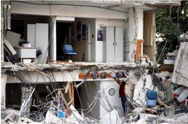
UN Office in Port au Prince after the earthquake
